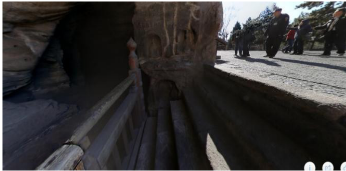
Figure 7 – The sinking place of the cave door
